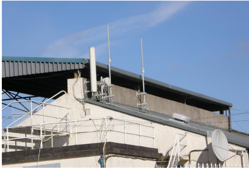
Transmitter Site Photo
